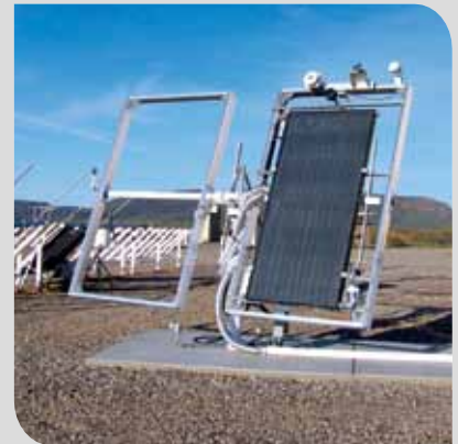
Dual Axis Solar Tracking Rack
